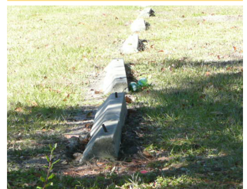
Poor overflow parking areas that could lead to an injury.
